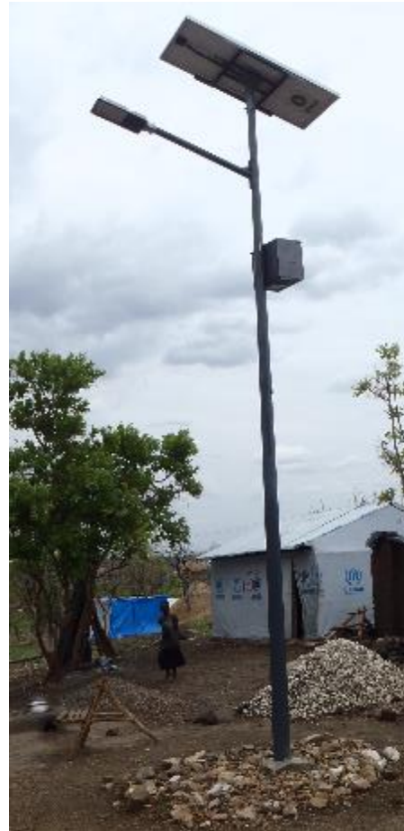
Photograph 1. An installed lamppost
