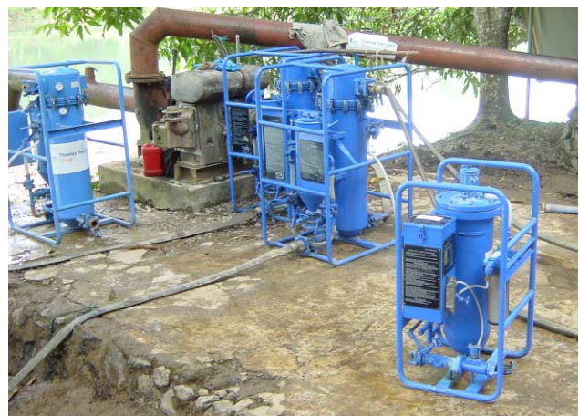
Figure 3 | Stella Meta Pre-Coat Filters in Operation in Aceh.
